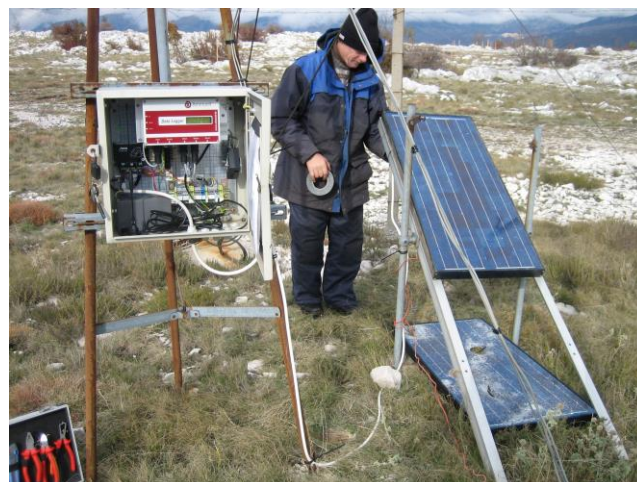
Fig. 5 Podvelez /SvetaGora - damaged solar panel
